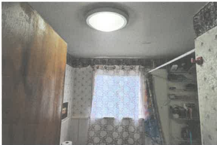
MOLD AROUND TOP OF WALLS.
