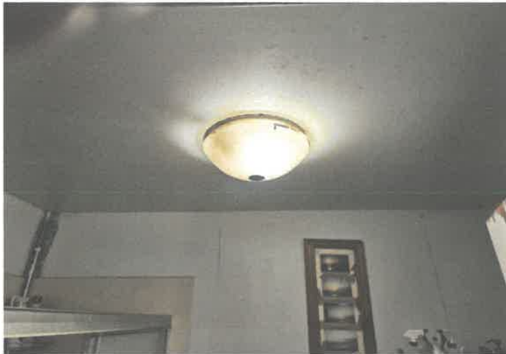
SEE MOLD IN CORNER OVER SHOWER.
